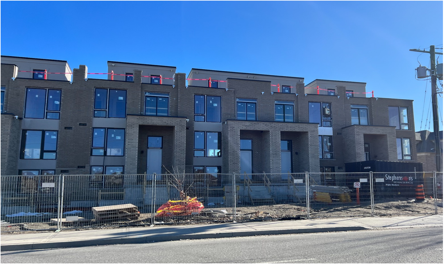
Photo taken on Feb. 26, 2024, showing the work done by the original construction team, before the receivership.
