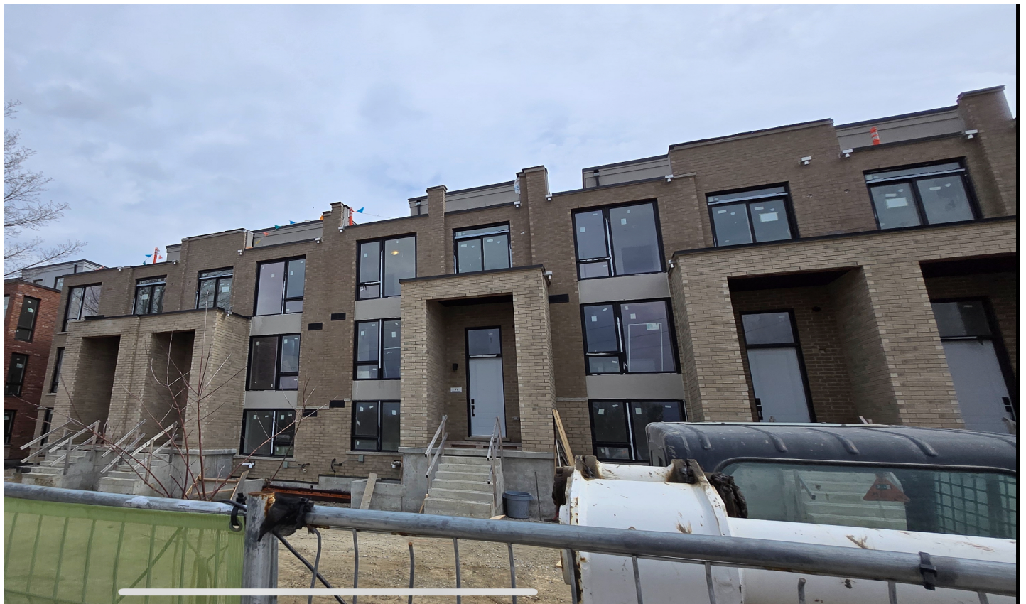
Photograph taken on April 29, 2025—16 months after the Receiver’s appointment—ironically showing no visible progress on the site. Railings remain uninstalled, and more critically, there is no safety protection in place. Ground refill has not started, far way from the claimed June 2025 completion. ( according to the original construction schedule, this block was to have been fully completed and delivered by April 2024.)
